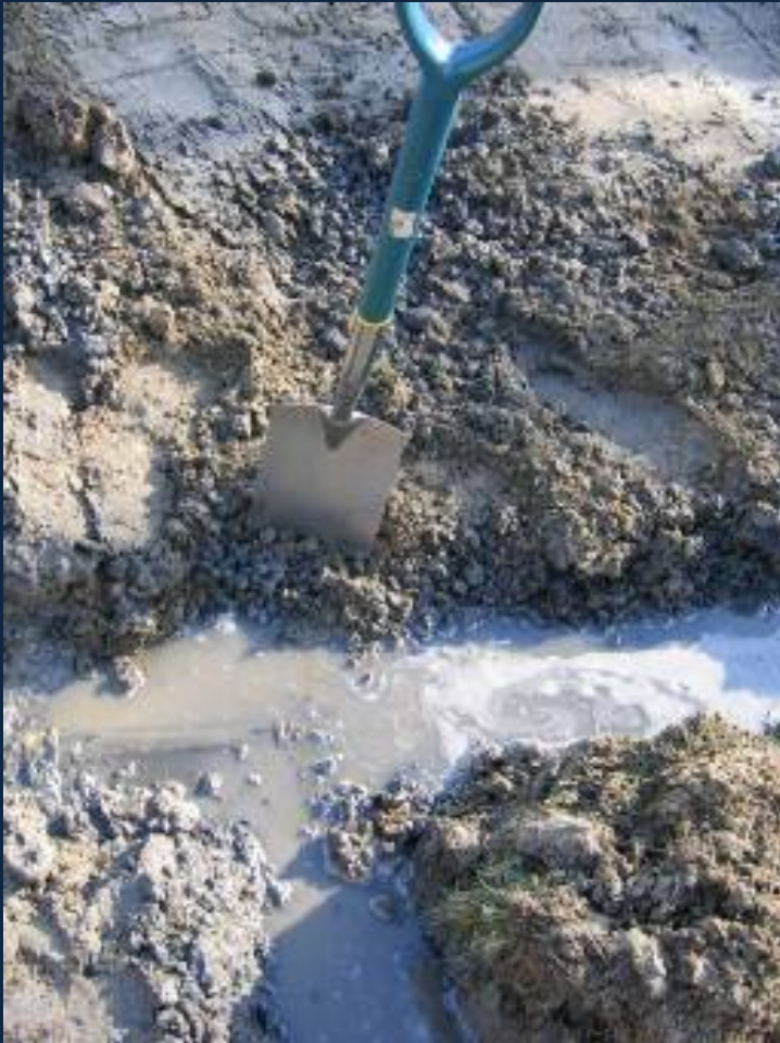
Ponding effluent above distribution pipes
