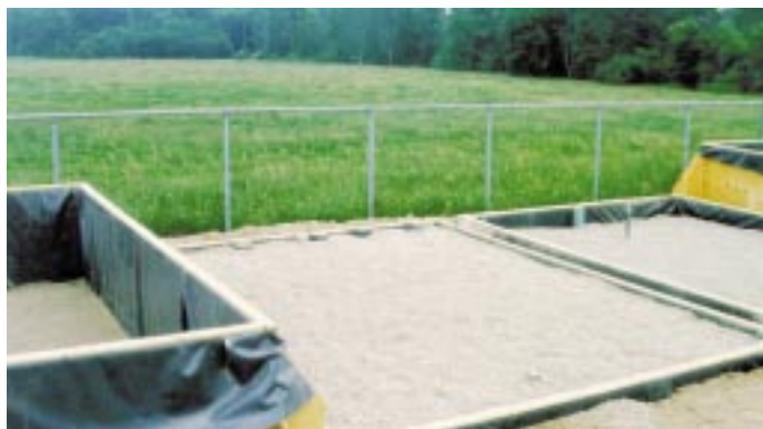
Close-up of four sand filters — Clifford, Ontario.
